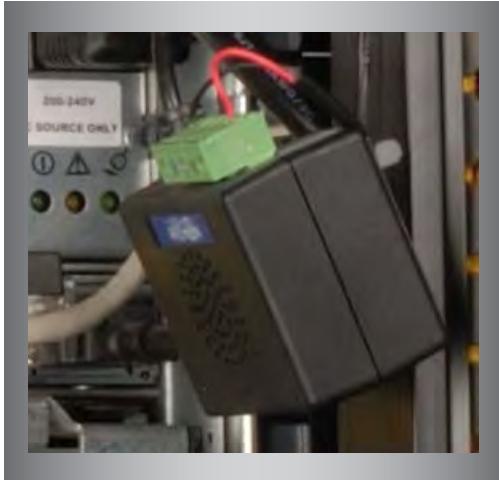
Use environmental sensors to monitor equipment intake temperatures remotely.
