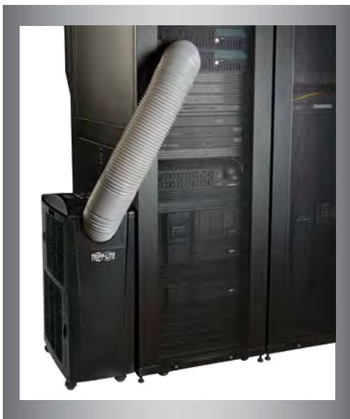
If heat-related problems persist, close-coupled cooling can be a smart and economical choice.
