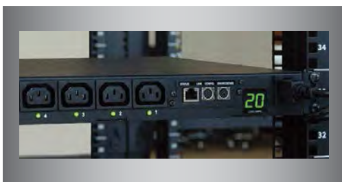
Load shedding uses switched UPS or PDU outlets to turn off non-critical loads during an outage.
