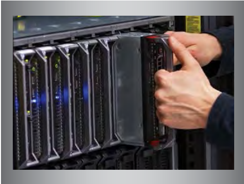
Blade servers and other high-density, high-wattage loads can create problematic hot spots if they're installed too close to each other.
