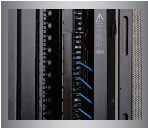
Cable management not only improves cooling efficiency, it also reduces troubleshooting time, repair time and installer errors.
